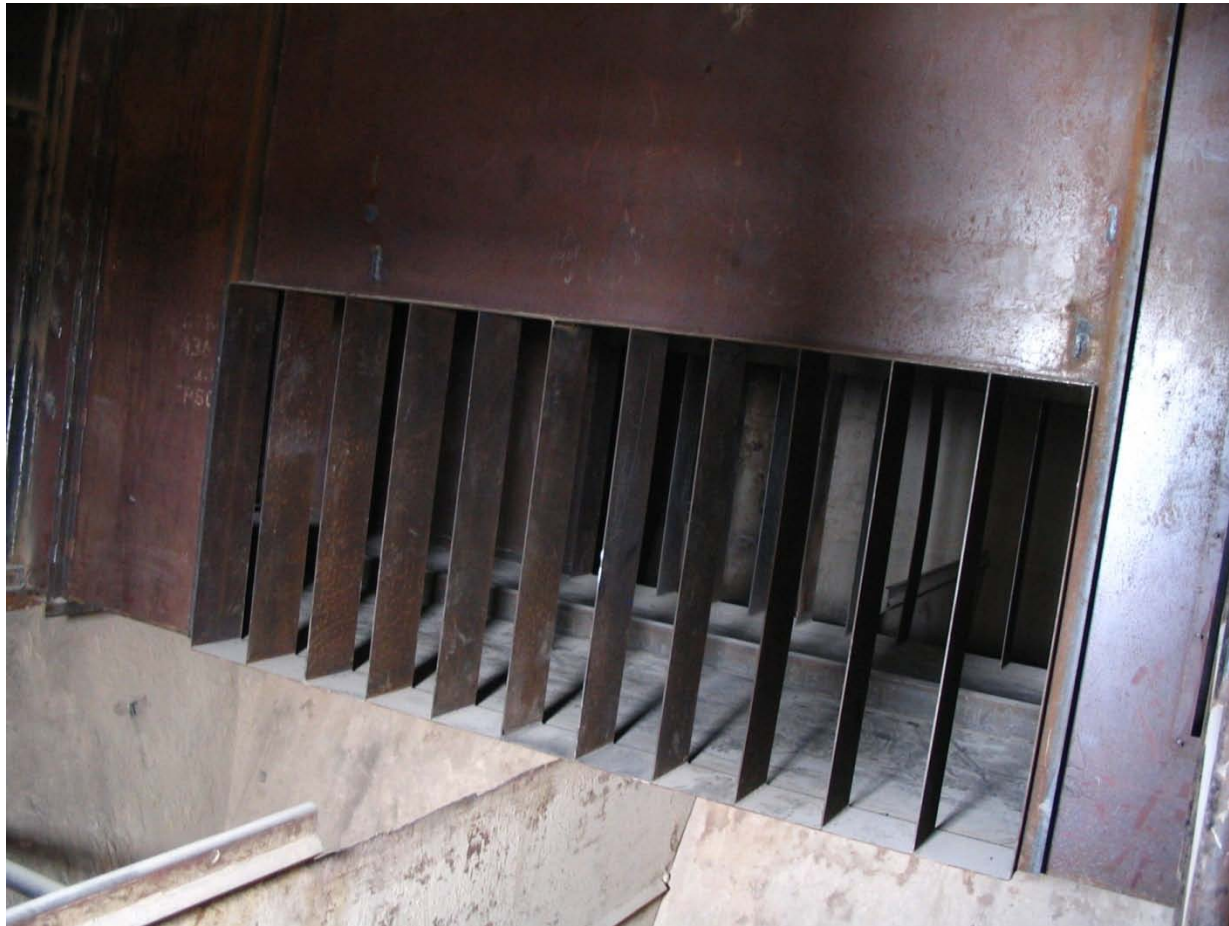
Inlet Plenum Vaned Compartment Entrance
