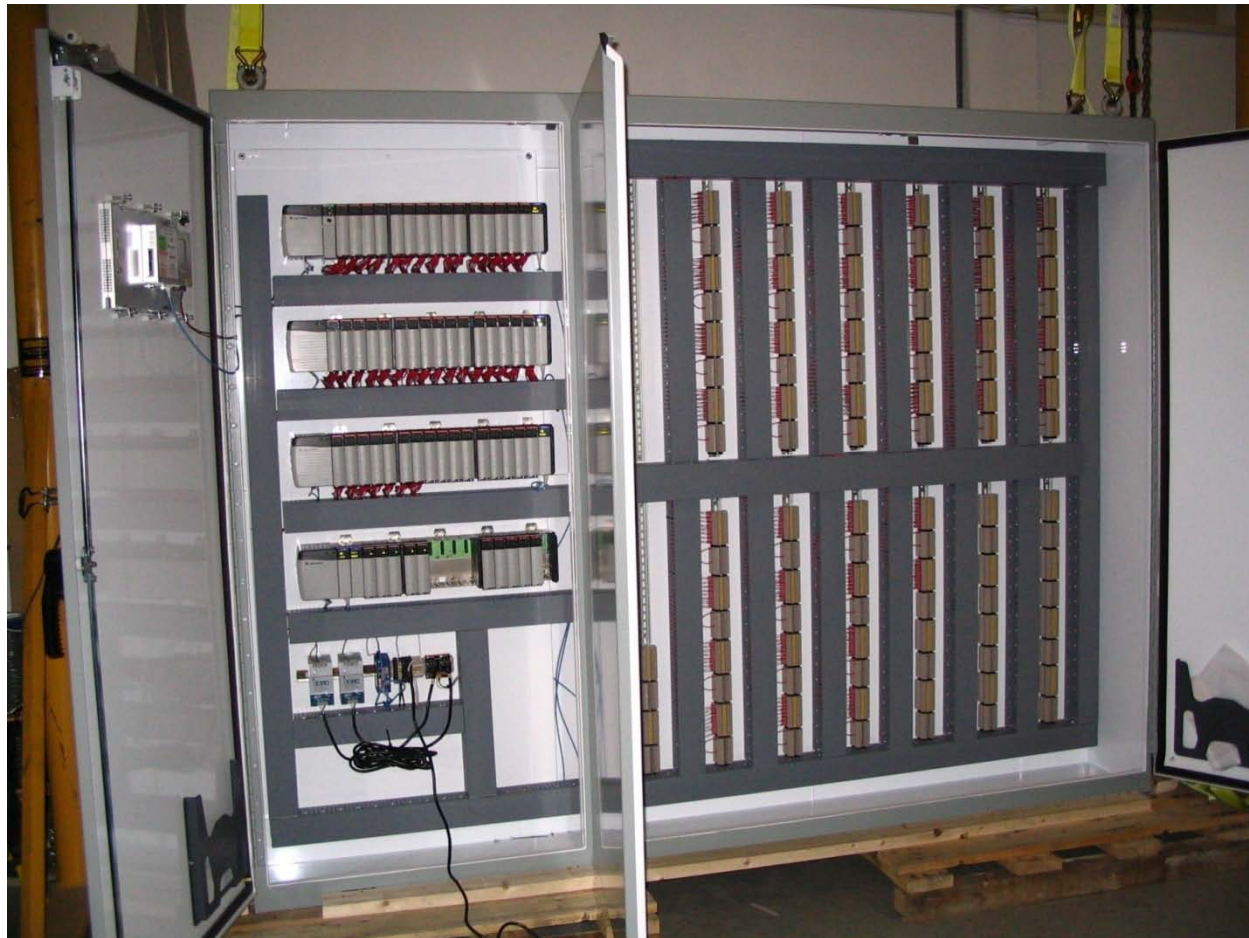
Big Stone Allen Bradley Logix 500 Control Cabinet
