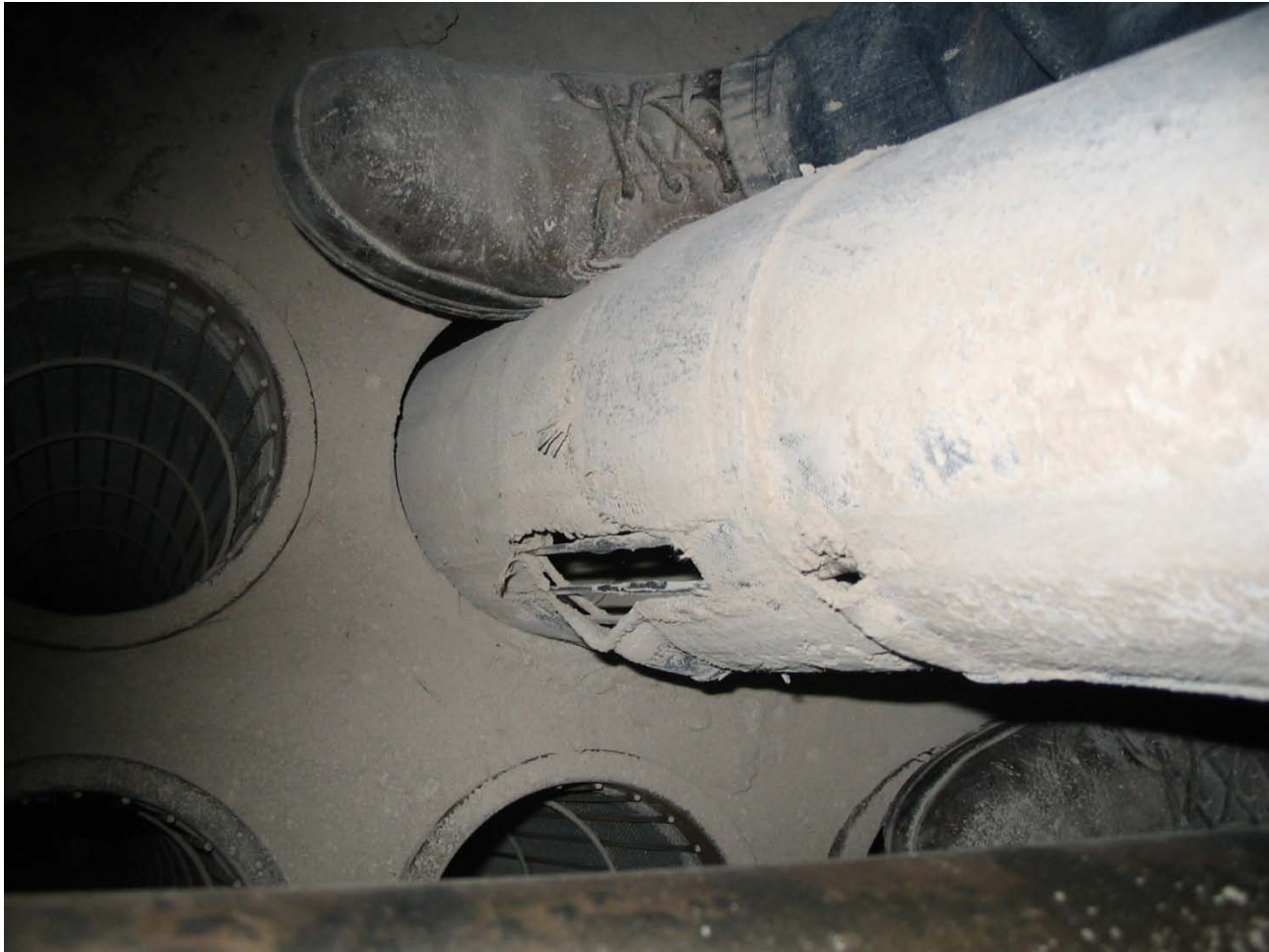
Bottom of Bag Failure due to Bags Touching
