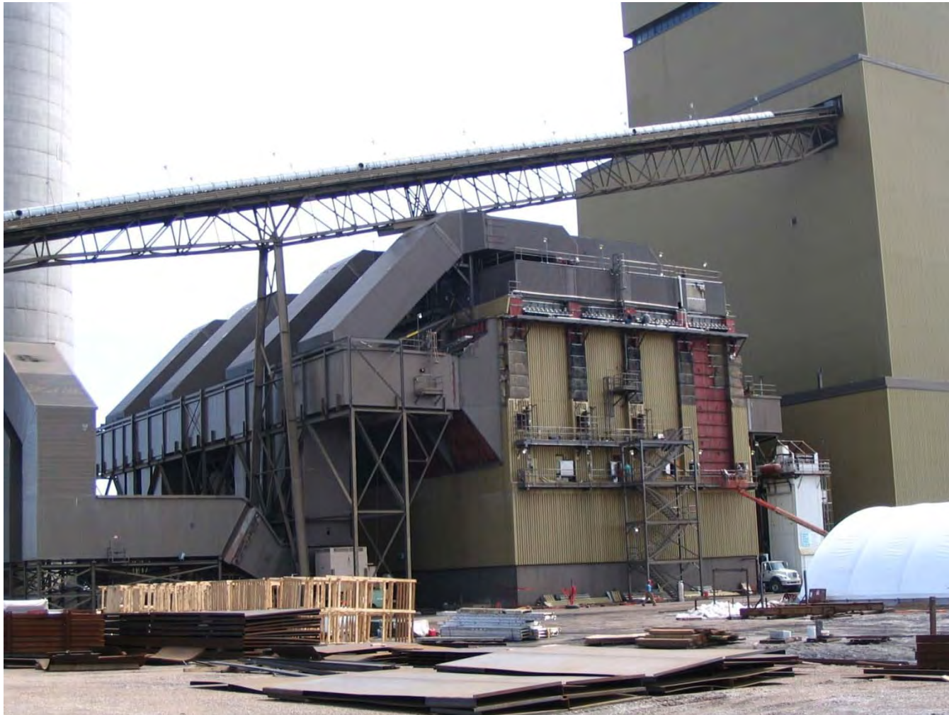
Big Stone Unit 1, Four Parallel ESP Chambers
