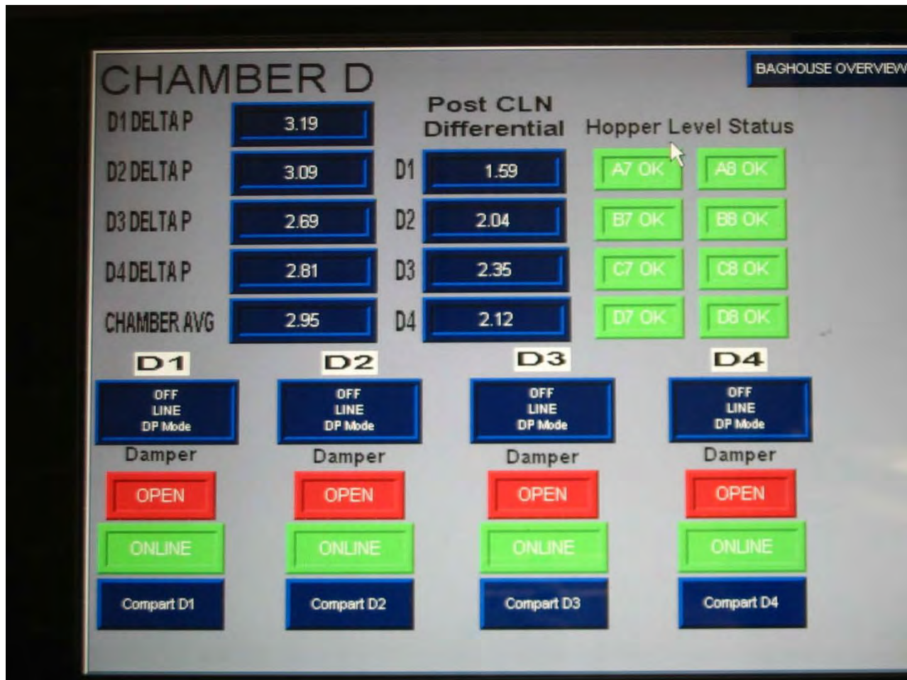
Control System Display Panel
